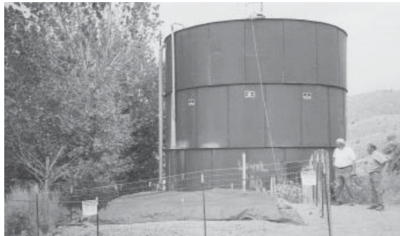
The "Little Red" 100,000 gallon tank failed in 1999.
